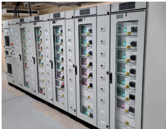
Figure 22: TGBT – Aéroport de Paris Orly.
