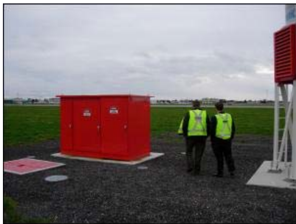
Figure 36 : Conteneur technique (source STAC)
