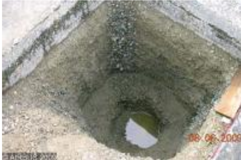
Figure 17 : Water contamination under the pavement
